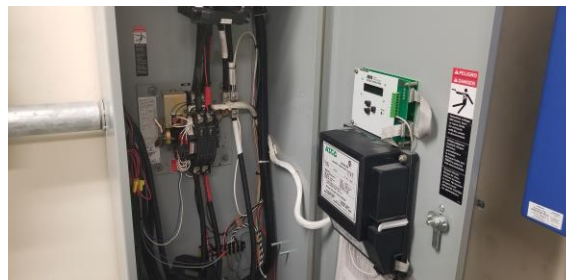
AUTOMATIC TRANSFER SWITCH (ATS)
