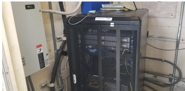
AUTOMATIC TRANSFER SWITCH (ATS)
