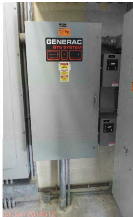
AUTOMATIC TRANSFER SWITCH (ATS)
