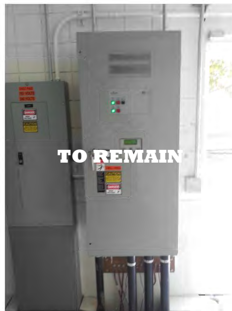
EXISTING AUTOMATIC TRANSFER SWITCH (ATS)
