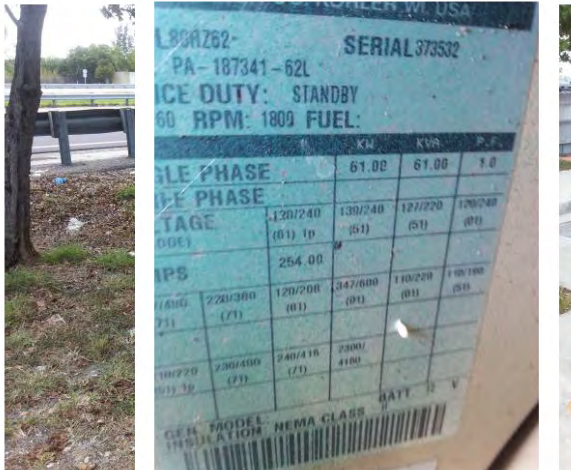
GENERATOR UNIT TAG
