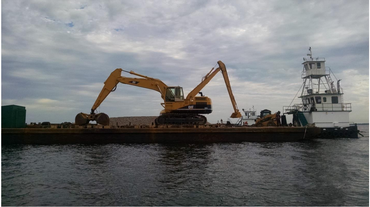
Figure 5: Heavy machinery used to deposit the oyster shell material from the barges onto the new reefs.
