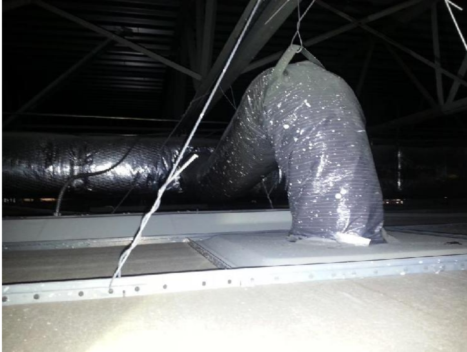
EXISTING MAIN SUPPLY DUCT AND FLEXIBLE CONNECTIONS
