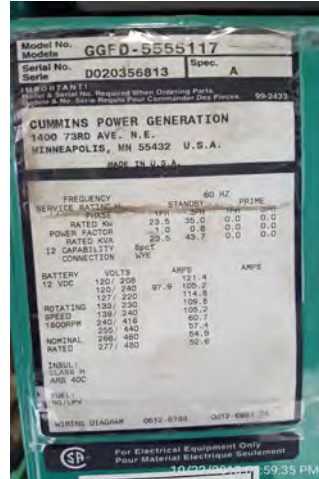
GENERATOR UNIT TAG
