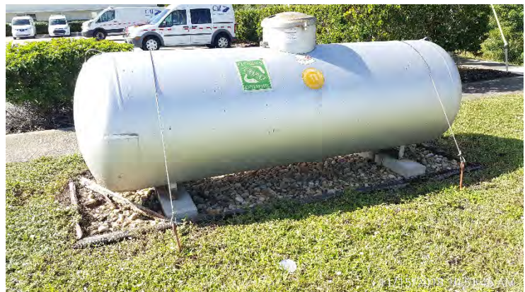
500 GAL. FUEL (LP) TANK
