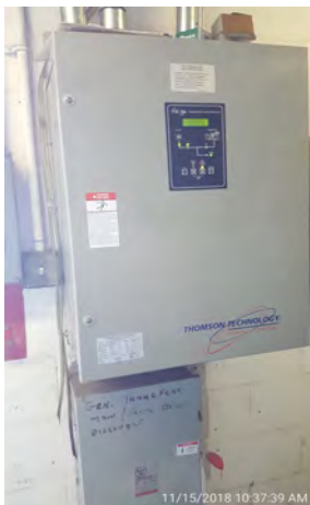
AUTOMATIC TRANSFER SWITCH (ATS)
