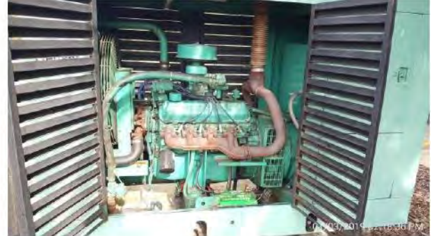
GENERATOR UNIT (INSIDE VIEW)
