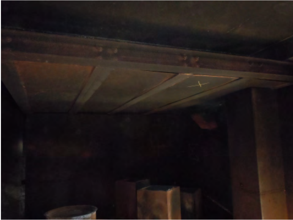
Photo #21 - Scenario Room #2 (NE) Ceiling Plates
