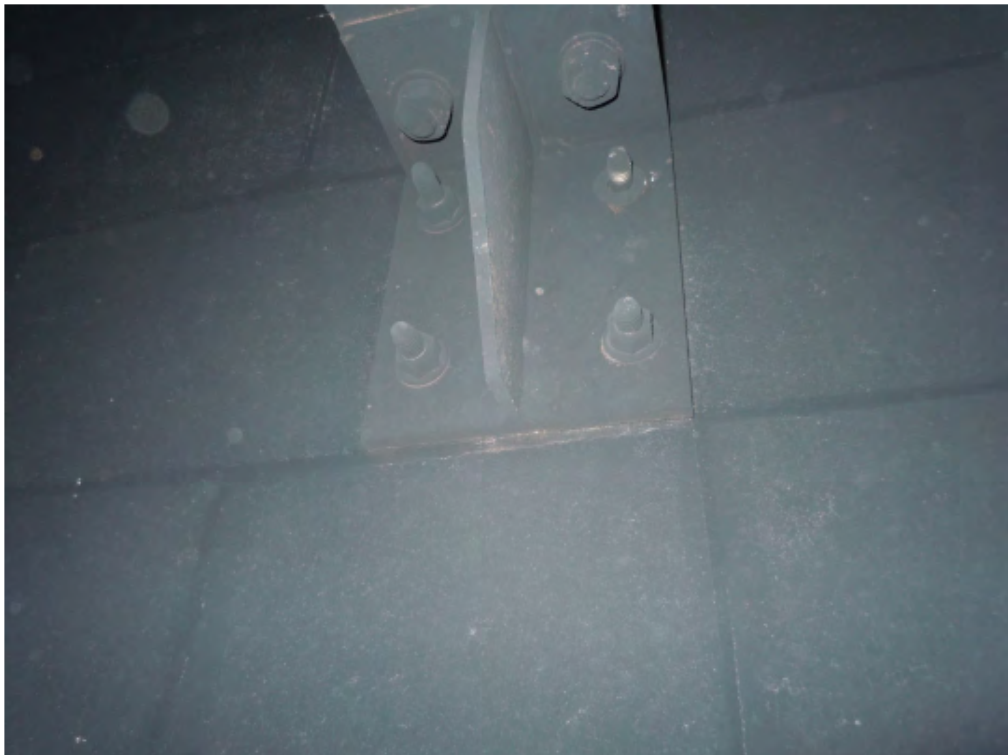
Photo #28 - Scenario Room #4 (SW) Missing Nut
