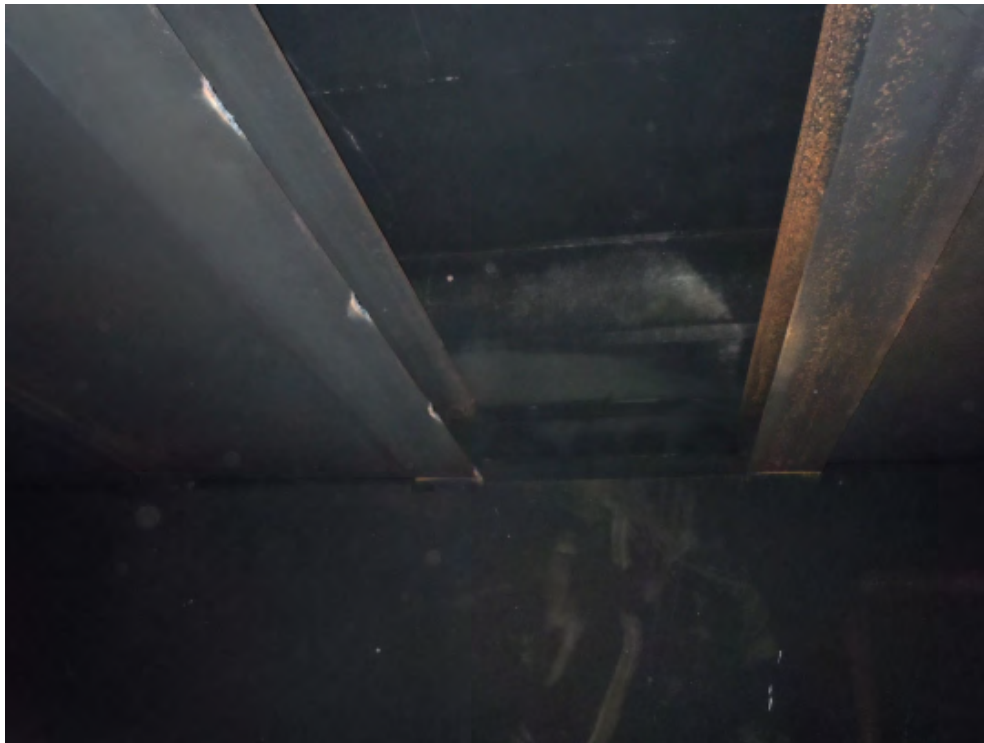
Photo #22 - Scenario Room #2 (NE) Ceiling Plate Removed
